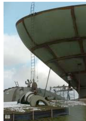
Summer opening: Work is done on the water tower at the FireKeepers Casino, which is expected to open in late summer.
